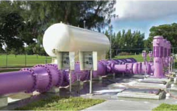
The color purple is used to identify pumps, tanks and pipes carrying reclaimed water for reuse. Photo courtesy of South Florida Water Management District.
