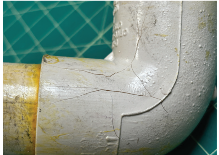
Photograph depicting a typical failure in a condensate-drain application
